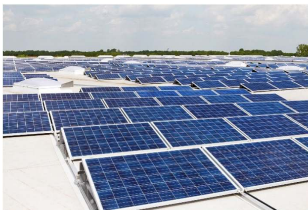
Fig. 1 Static Solar Panel (Picture from Internet)
